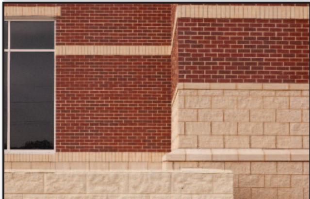
Multiple colors of brick as well as split face and ground face block combine to create a pleasing presentation for this massive structure.
