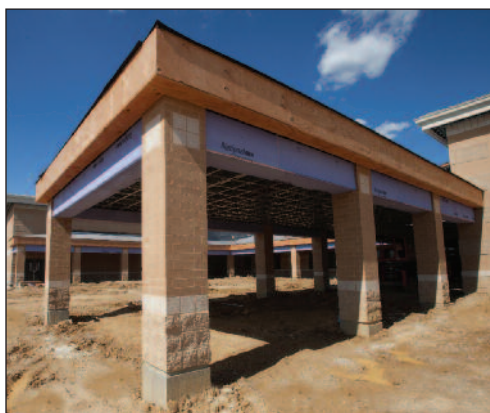
THE DOUBLE WINGED CANOPY AND COLONNADE UNDER CONSTRUCTION SHOWS THE USE OF SPLIT FACE AND GROUND FACE BLOCK AS WELL AS UTILITY BRICK ON THE COLUMNS.
