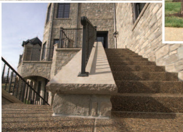
ABOVE: SMOOTH FACED AUXVASSE LIMESTONE CAPS ARE PART OF THE EXTERIOR STAIRWELL WALLS AND PROVIDE A SOLID BASE FOR HANDRAILS. PHOTO BY CREATIVE EDGE.
