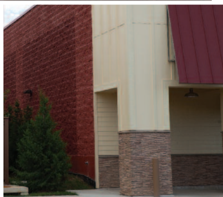
THE CHOICE OF LOAD BEARING MASONRY WALLS WORKED WELL IN THE TIGHT CONSTRUCTION SITE ON A CORNER LOT AT A BUSY INTERSECTION.
