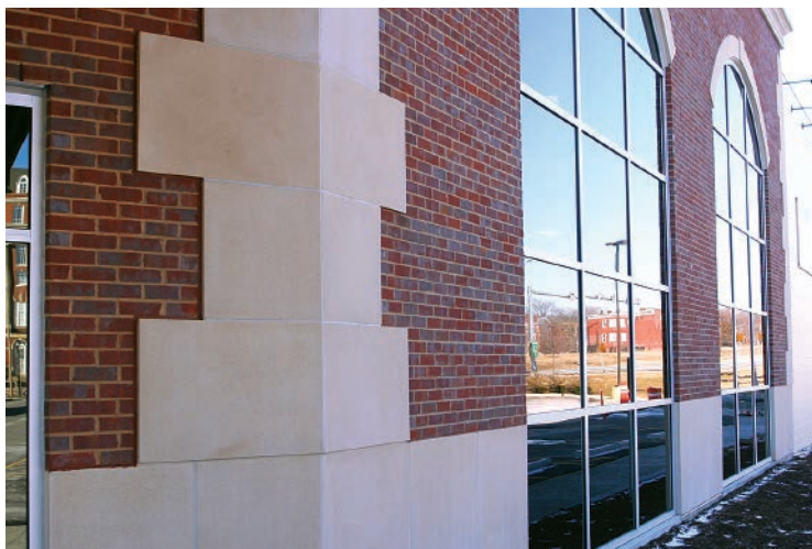
CAST STONE QUOINS, ARCHES AND VENEER BRICK REFLECT MASONRY DETAILING IN THE SURROUNDING NEIGHBORHOODS.
